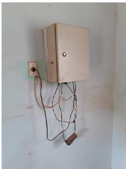
Painel de controle
