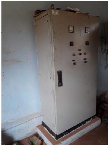
Painel de controle
