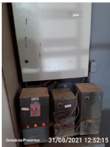
Painel de controle
