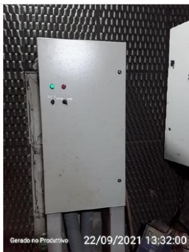
Painel de controle
