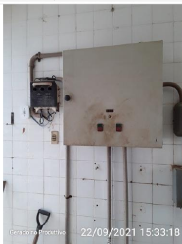
Painel de controle
