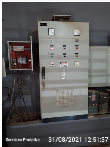
Painel de controle
