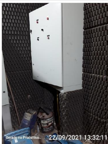
Painel de controle
